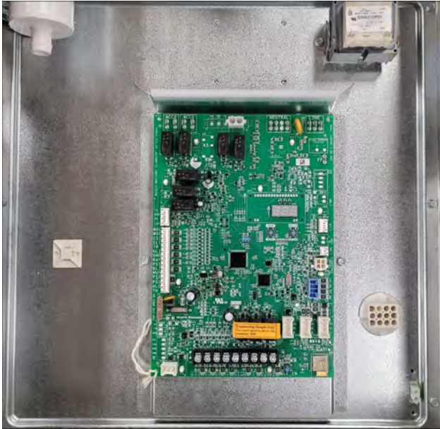
Figure 37. IFC and blower vestibule
